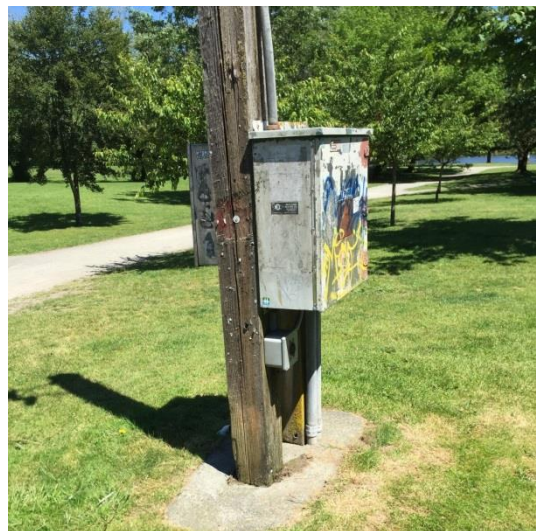
Figure 5 (above): Photo of anticipated connection point to BC Hydro electrical system at Trout Lake (facing northeast). Electrical supply at this location will require upgrades to supply more power to support EV charging infrastructure
