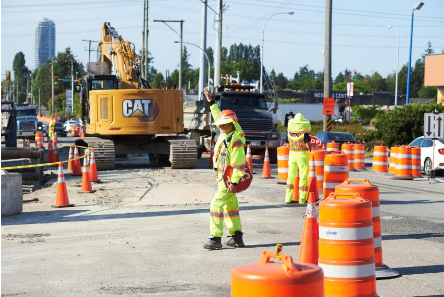
Traffic control personnel working at Kennedy Newton Water Main – Scott Road Section
