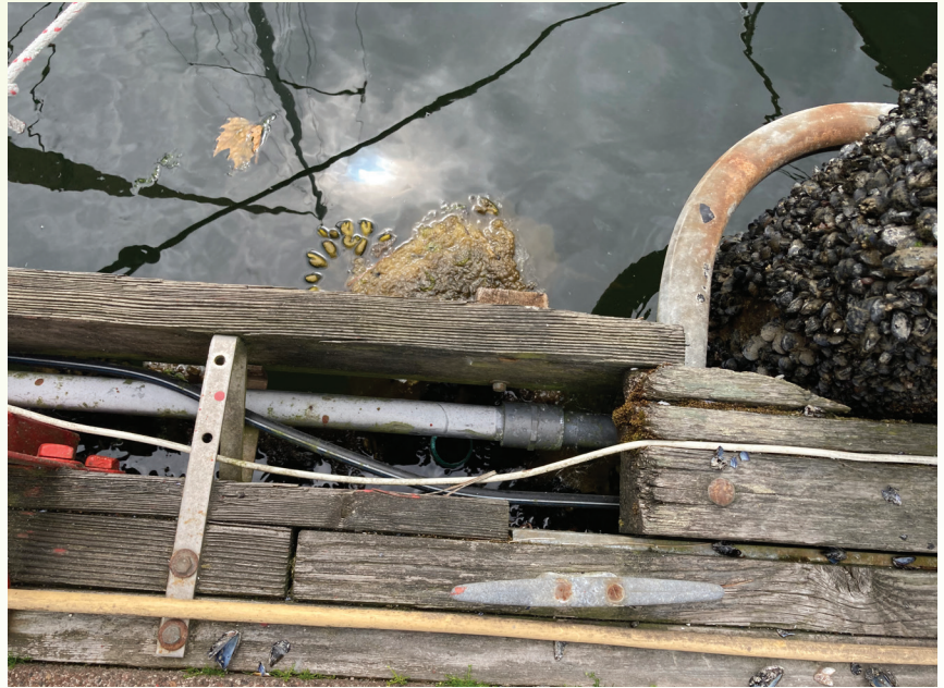
Wooden dock and plumbing infrastructure at Heather Civic Marina
