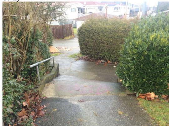
Stair and hedge condition east side
