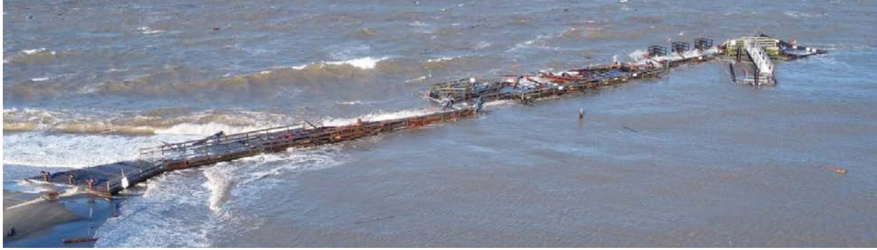
Fig. B: Deck inundation during Jan 2022 storm
